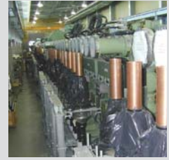
TERMINATIONS READY FOR CONNECTION TO MAIN CIRCUIT TERMINALS
